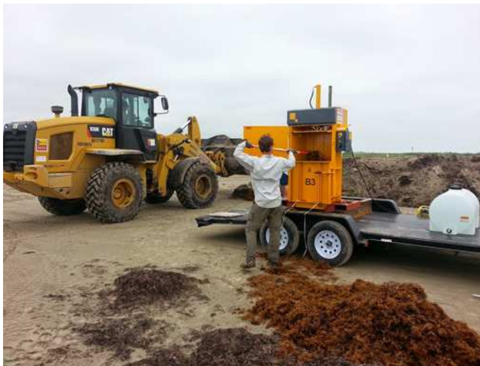
Figure 2.4: Photo of dune construction and seabaling operations. The dune was constructed using heavy front-loaders.
